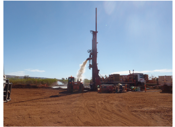
FIGURE 5 A A DRILLING RIG DRILLING FOR A DEWATERING BORE. AIR FROM A LARGE AIR COMPRESSOR IS INJECTED INTO THE HOLE BELOW THE AQUIFERS LIFTING WATER OUT OF THE HOLE.
